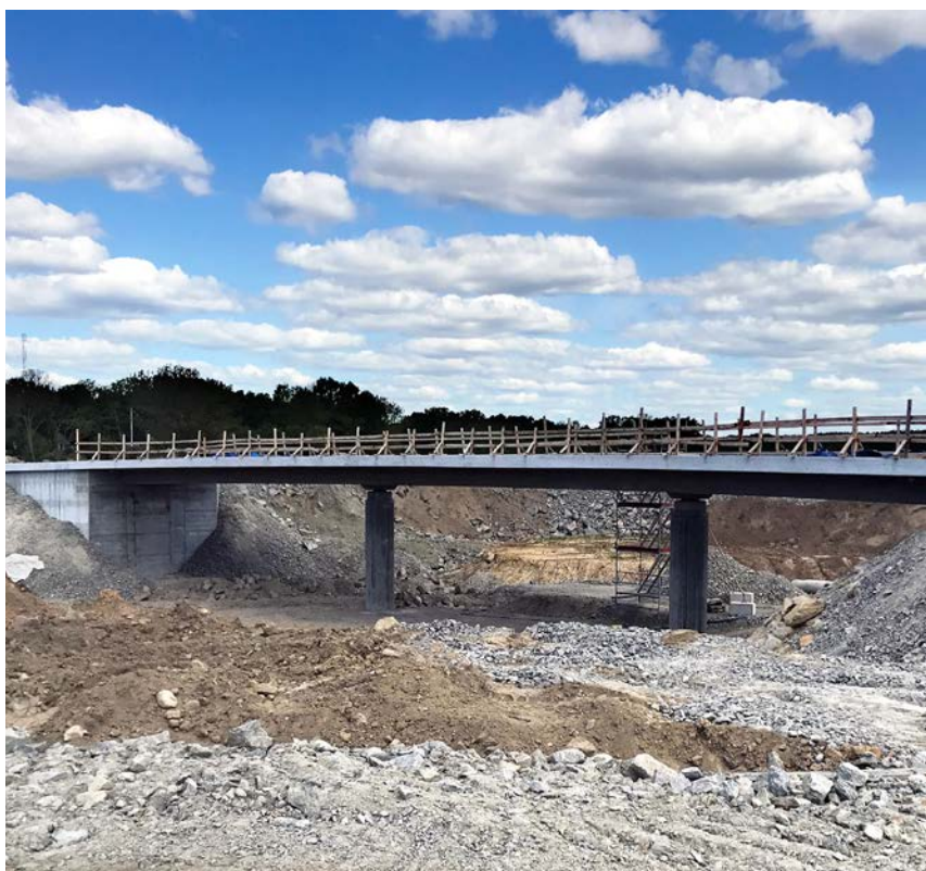
One of the 23 bridges being built to enhance infrastructure, where Leca LWA prevents additional piling.
