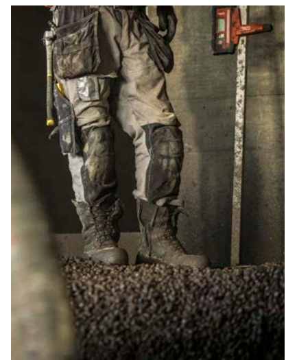
3,500 cubic meters of Leca LWA have been delivered, used both as insulation material between floors and as fire protection
