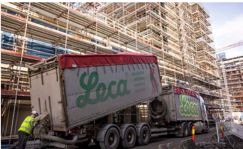
It is quick and easy to install Leca LWA compared to alternatives like polystyrene, which would require extensive use of construction cranes and more manpower.
