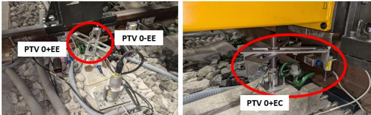
Figure 84.- Detail of the potentiometers used to measure the vertical displacements of the under-rail pad
