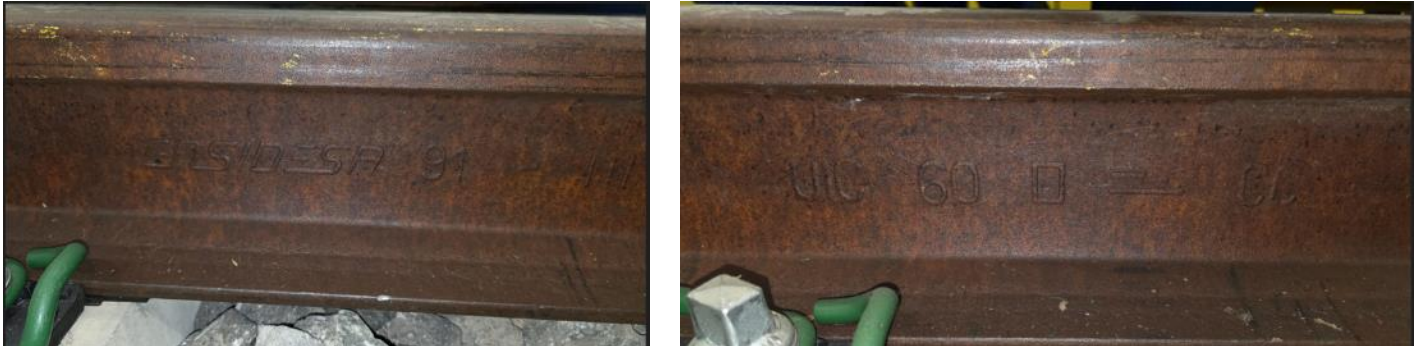
Figure 17: UIC 60 rail used in railway track section
